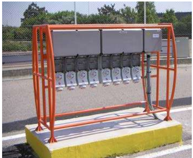
Container Terminal, Le Havre – France
