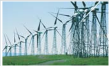
Wind Power station
