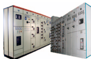
Series of electrical controlled equipment area
