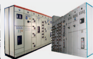
Series of electrical controlled equipment area
